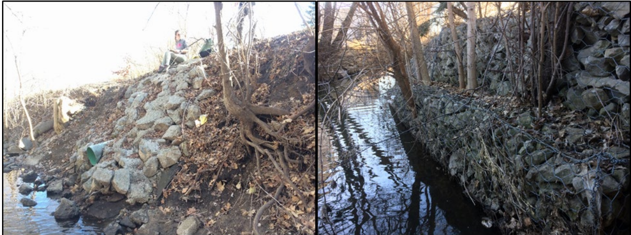
Figure 46. The image on the left shows a poor example of bank stabilization, where debris and cement was slopped into the stream and down the bank. Concrete is not a good way to stabilize it gives no movement for the stream and will speed up the waters movement causing more erosion to occur. The image on the left is between UNI's campus and College Street where apartments are being built, these apartments are right on the streams edge and rip rap was implemented to control bank erosion throughout this area. This kind of stabilization will help to prevent erosion, but not allow the steam to move at all.
